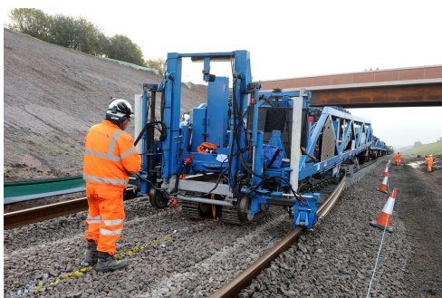
Specialist track laying equipment at Norton Bridge – as part of the laying of 10Km of new track
