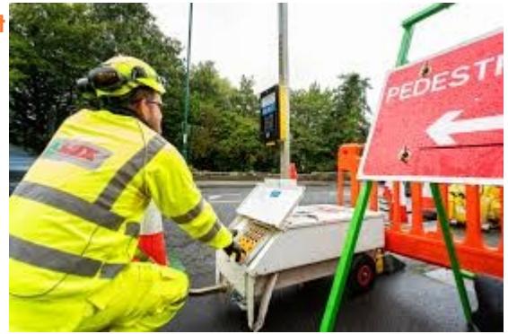
The safety of all road users needed to be taken into account, which lead to revised schemes
